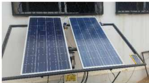
Fig. 15. Two-string photovoltaic generator with reference cells.
