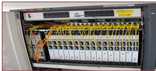
Optical Line Terminal "OLT"
