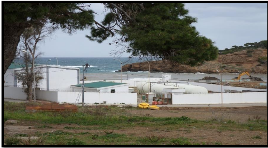
Figure 49 - Station de Pompage ( Honaine)
