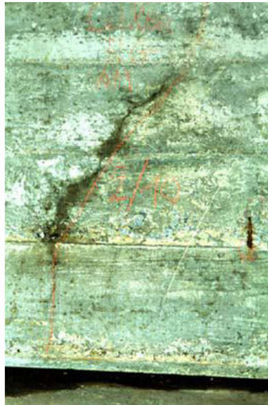
Figure I.1: Exemple de fissuration
