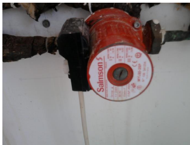
Figure II.14 : Pompe de circulation TYPE SALMSON [69].
